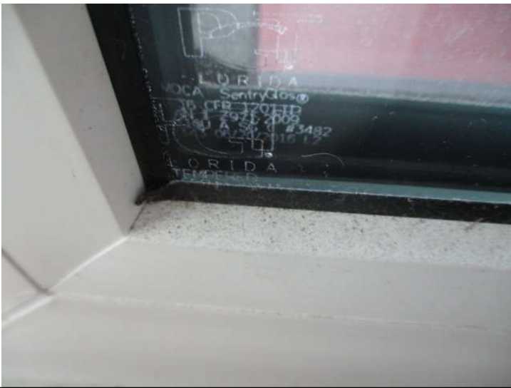
Exterior Opening Protection
